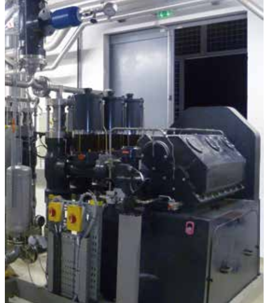
Autoclave feeding, using single-acting FELUWA MULTISAFE® double hose-diaphragm pump in triplex configuration.
